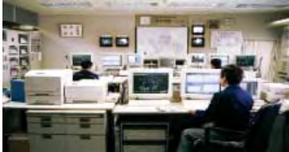
Centralized monitoring and control room
